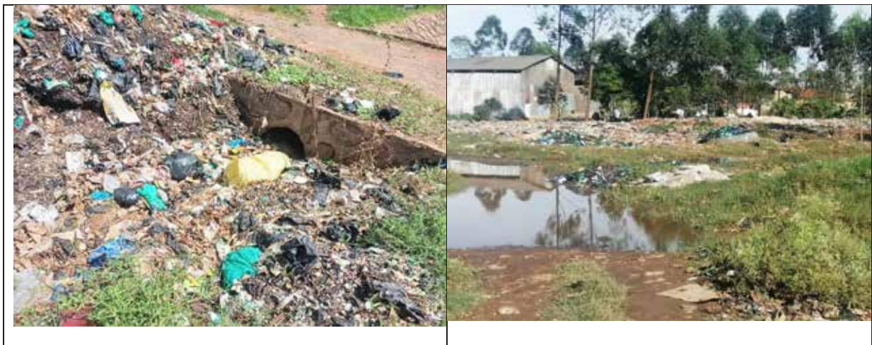
Figure 7: Illegal solid waste dumping in a drainage channel in Gombe division and on open bare ground
